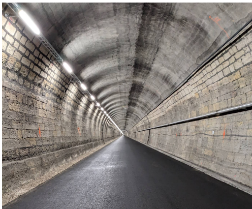
Figure 5. View inside the tunnel. On the wall the natural stones are shown, the tunnel ceiling is covered in sprayed concrete, and the floor is tarred.
