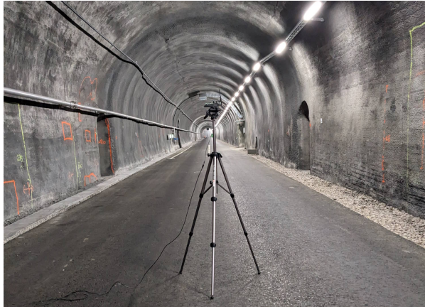
Figure 7. Data-Logger during measurement in the middle of the tunnel. The tunnel walls and ceiling are covered in sprayed concrete
