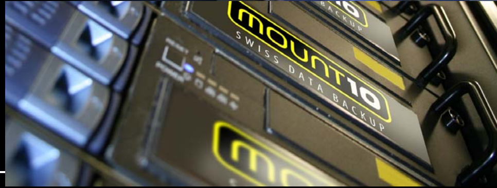
Swiss High Security Data Center (i.e. Mount10)
